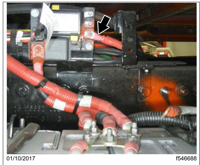
Fig. 29, CPDM Power Cable on the PNDB
