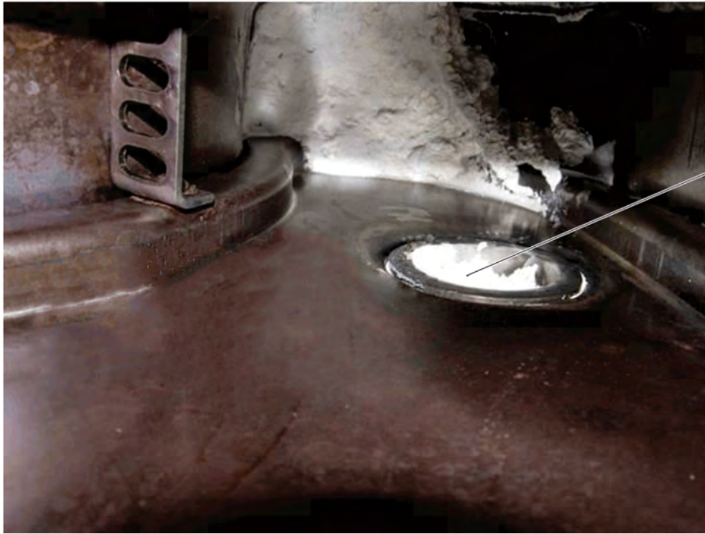
Looking inside SCR Mixing Chamber with DPF removed. Note: Doser Port Location
