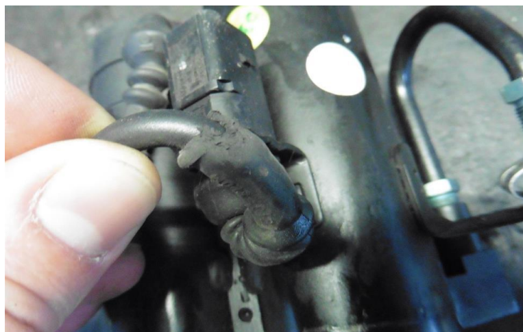
Figure 1. Damaged insulation on the electric cable for the shock absorber.
