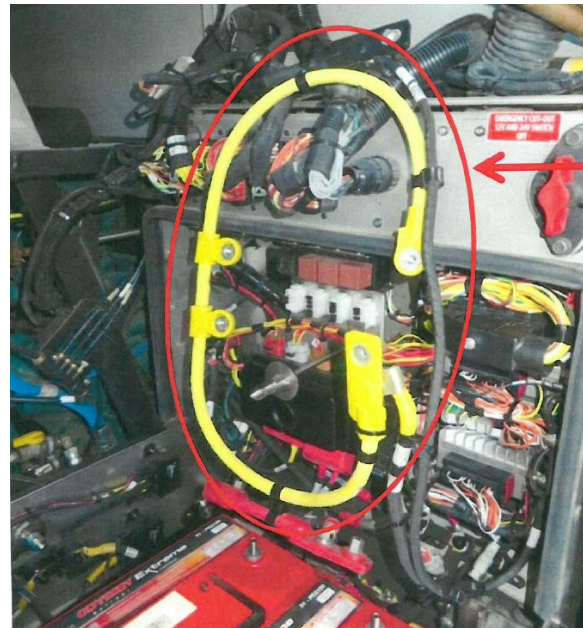
Figure 19: SECURE UP CABLES
