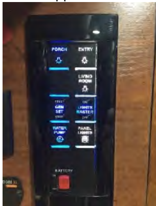
Kitchen Upper End Panel Switch
