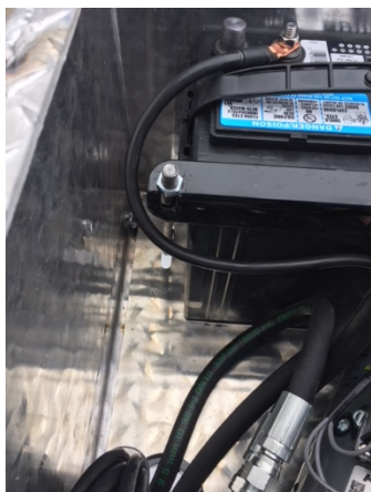
No Ground Wire
