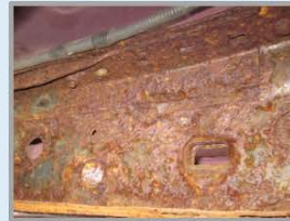
Complete Surface Rust with Descaling
