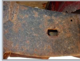
Light to Moderate Surface Rust
