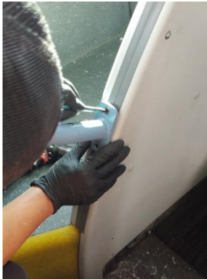
Figure 16: Mark Stanchion Holes
