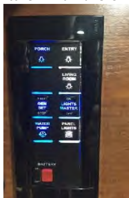
Kitchen End Panel Switch
