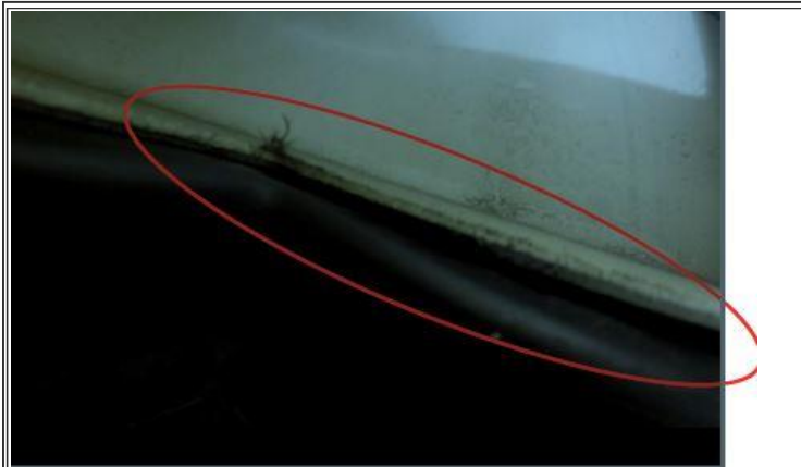
Figure 1: Gap between Boot seal and Hood
