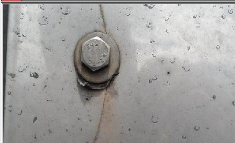
Figure 1: Heat Shield crack
