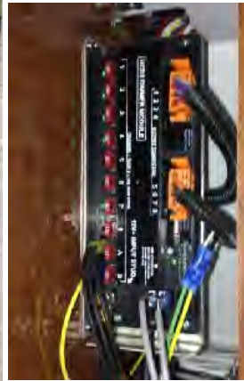
Kitchen upper fuse panel
