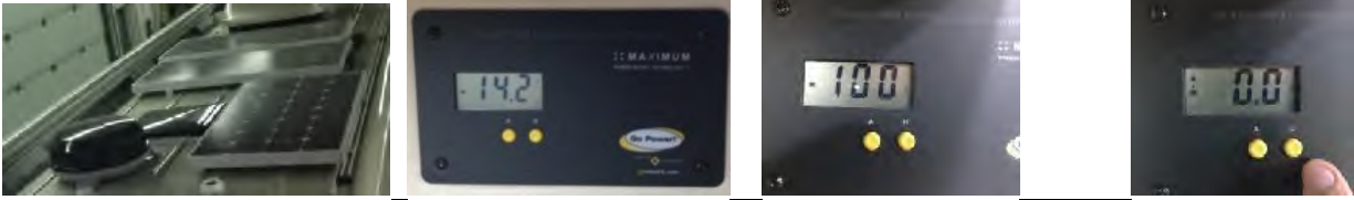
(Shown with three panels 285 watts) (Battery Voltage) (Battery Charge condition) (Solar Charge Rate)
