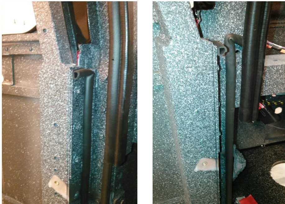
Front door seals
