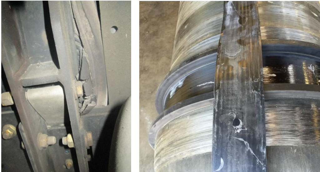
Figure 2. Worn and displaced rubber isolators under the J-bracket in a 237-series side mount system.
