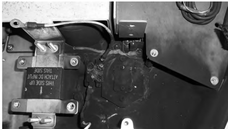
Figure 15. Smoke Damage Caused by Failed Passive Discharge Resistor – NOT REPAIRABLE
