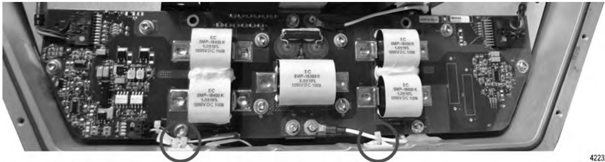
Figure 6. HVIL Circuit Card – Two (2) Wire Tie Locations
