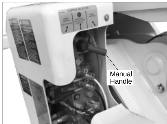
Figure 2 — Original Manual Valve
