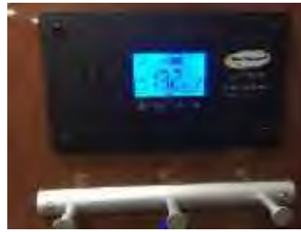
Display panel next to the main entrance door
