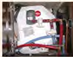
Summer Position / working water heater
