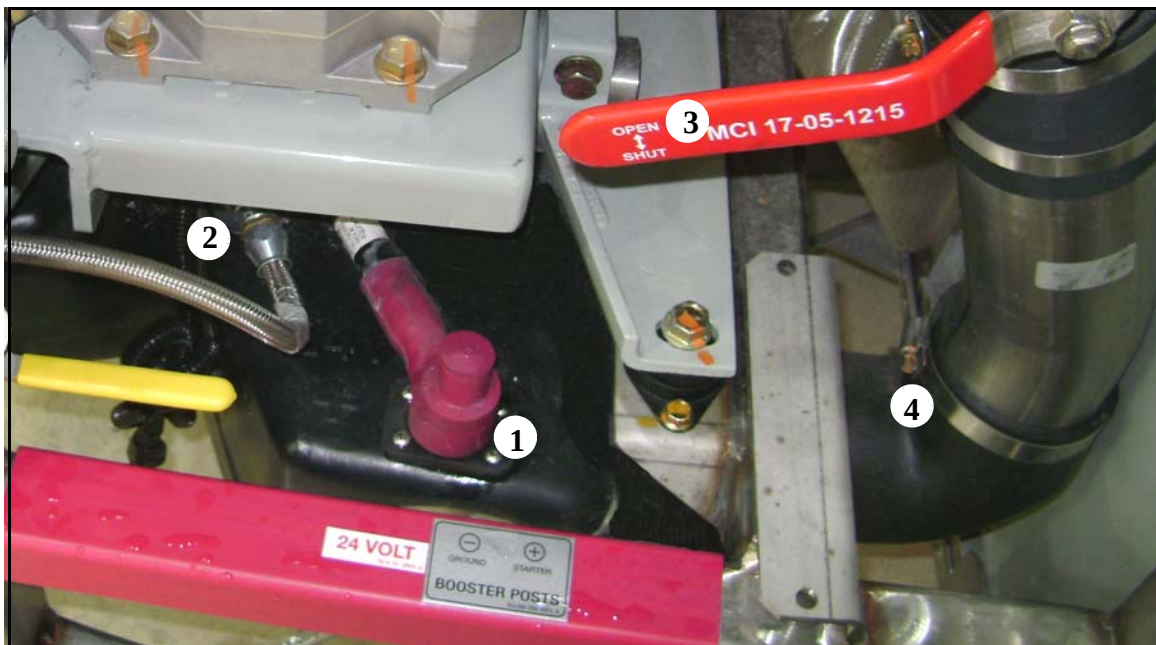
Figure 25. Secondary, lower lavatory tank assembly.
