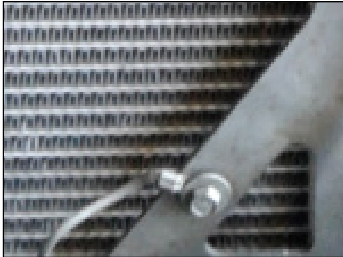
Figure 14 - Typical View of Ground Cable Connection
