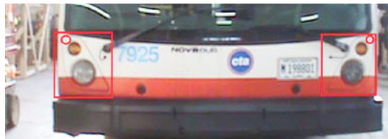
Figure 50 - Install the Turn Signals and Headlights
