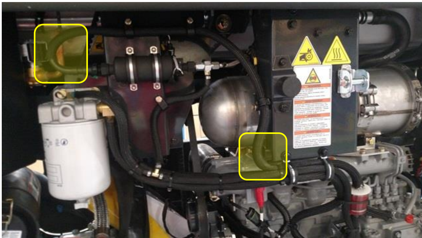
Figure 7: Picture of bypass installation. Insure highlighted areas are not kinked.
