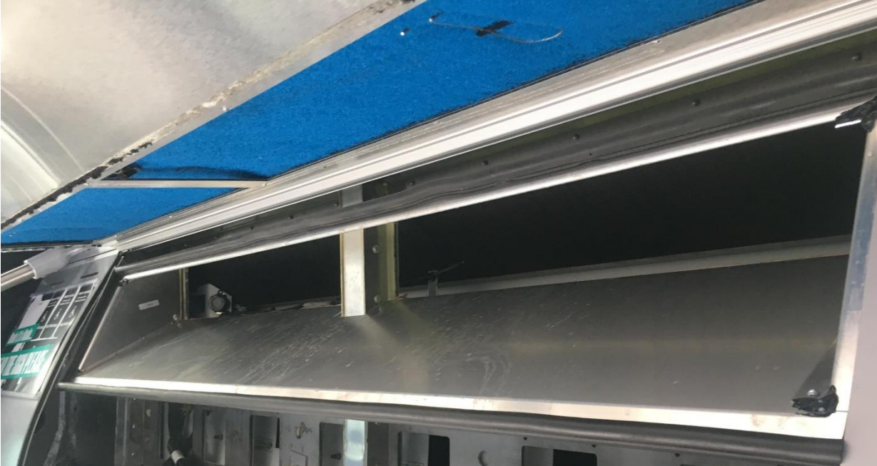
Figure 4: Bulb seal on edge of return air ducts
