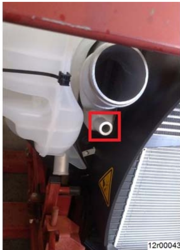
Figure 1, Air Compressor Inlet Tube Port on Charge Air Cooler Causing Water Ingestion.
