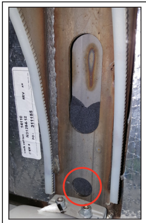
Figure 7 - Typical View of Hole and Cut-out covered with the Large Foam Piece
