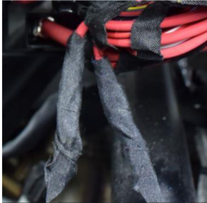
Figure 30. Original power wires.
