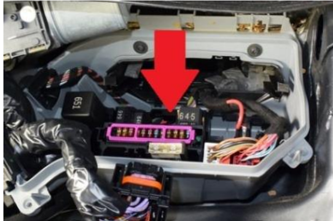
Figure 4. Fuse panel B -SB- in the E-box
