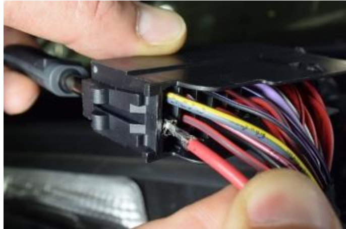
Figure 14. SB1 battery power feed wire.
