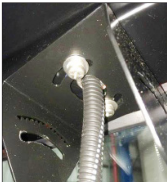
Figure 3 - New Washers and Thread Locker Added
