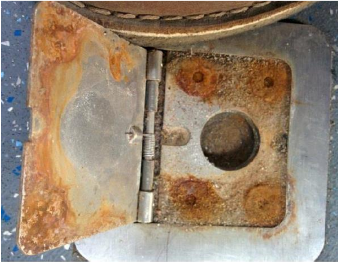
Typical Floor Plate Hardware Rusting
