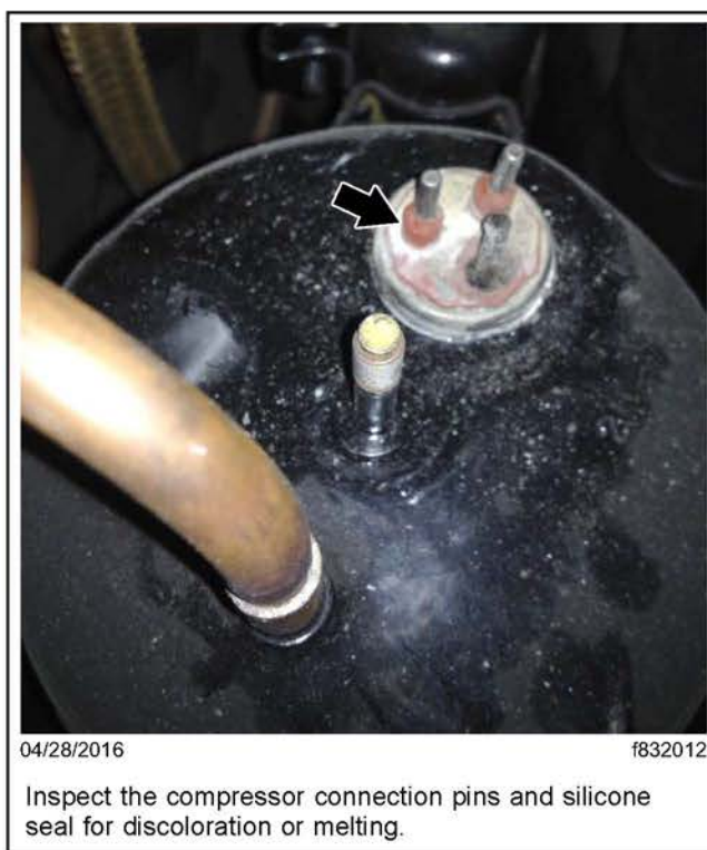
Fig. 11, Melted Silicone Insulator and Compressor Pin Damage
