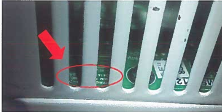
Figure 2, Looking at FET Board thru grill
