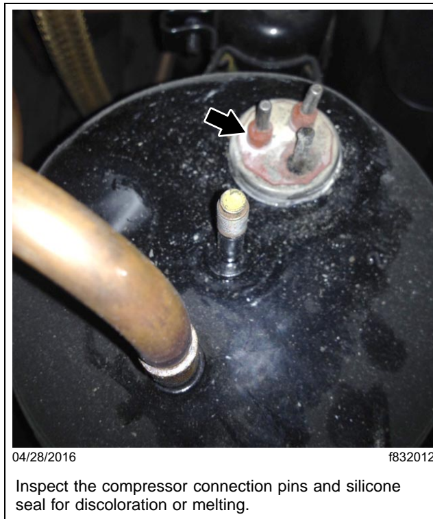
Fig. 11, Melted Silicone Insulator and Compressor Pin Damage
