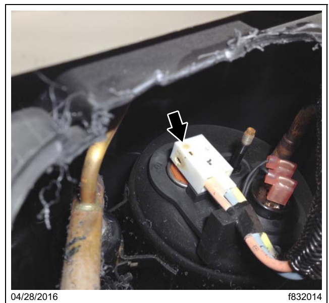
Fig. 8, Yellow Discoloration and Melting of the Block Connector
