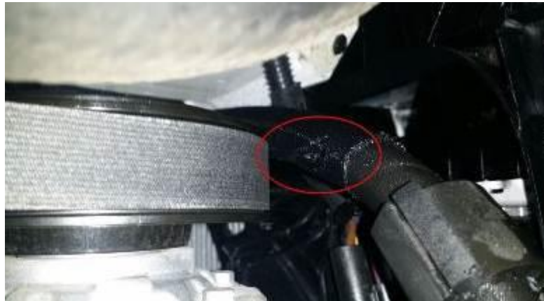
Figure 1. Point of hose contact with air conditioning compressor pulley.
