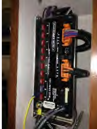
Kitchen upper fuse panel
