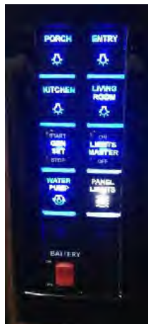
Kitchen End Switch Panel
