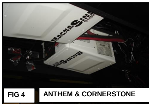
Fig 3: Anthem / Cornerstone inverters are located in 3rd compartment forward of rear wheels on either side .
