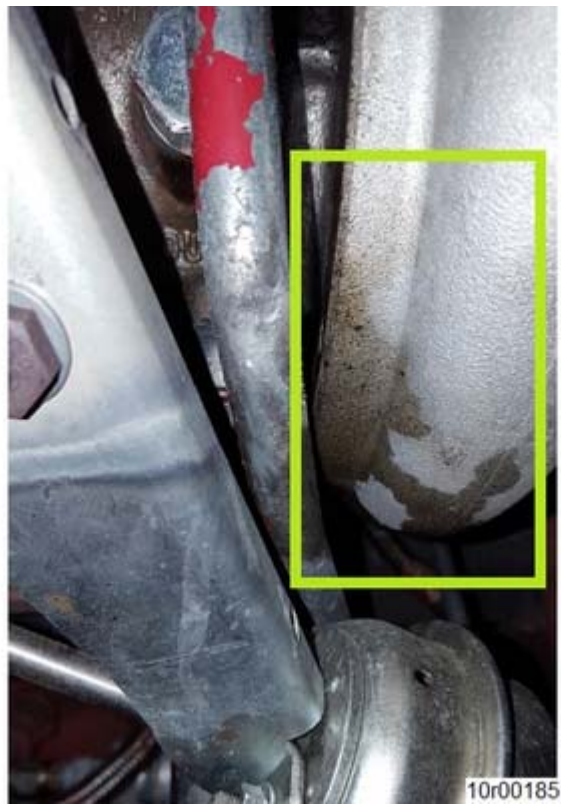
Figure 2, Class 2 Oil Leak.
