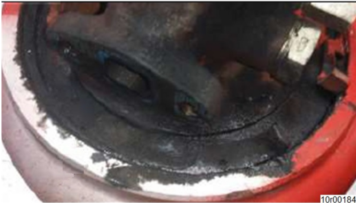
Figure 1, Class 1 Oil Leak.
