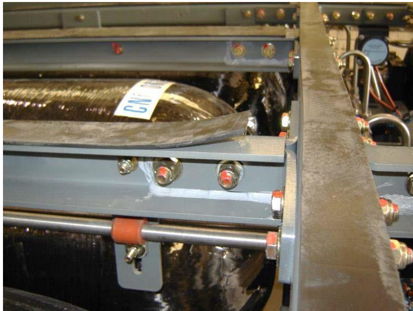
Figure 2 Mounting surfaces must be cleaned, new adhesive and rubber strips applied as needed.
