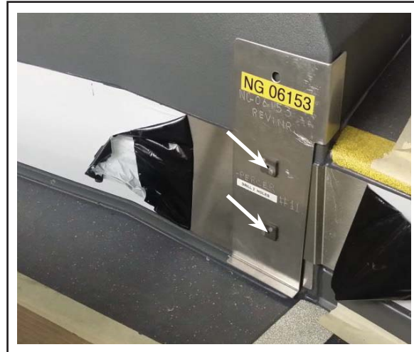
Figure 3 - Drilling Two Holes with NG06153 Drilling Jig in Street Side Wheelhouse Kick-Plate
