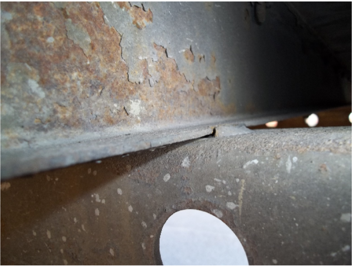
1 BROKEN CROSSMEMBER TO SLIDER RAIL WELD
