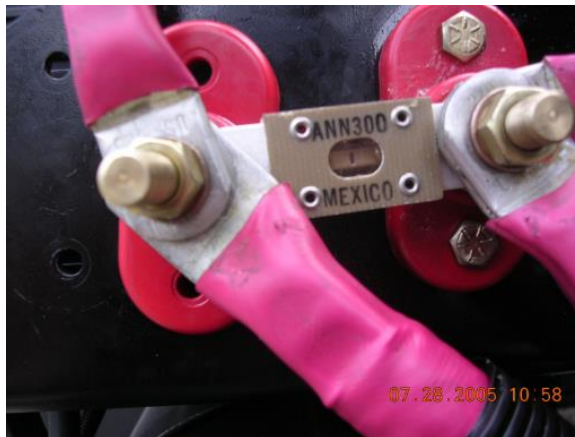
Example of 300 Amp Fuse
