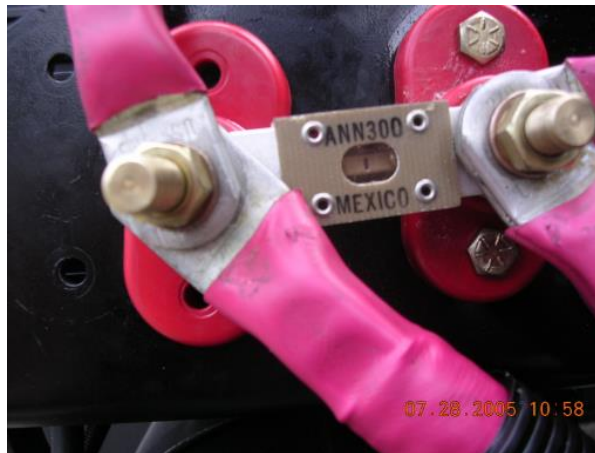
Example of 300 Amp Fuse
