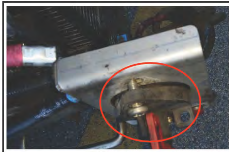
Figure 4 - Loosening of Main Battery Disconnect Switch
