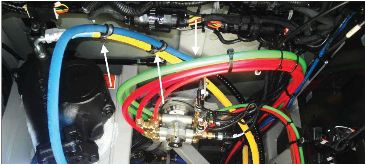
Figure 4: P-clamps in front service compartment.
