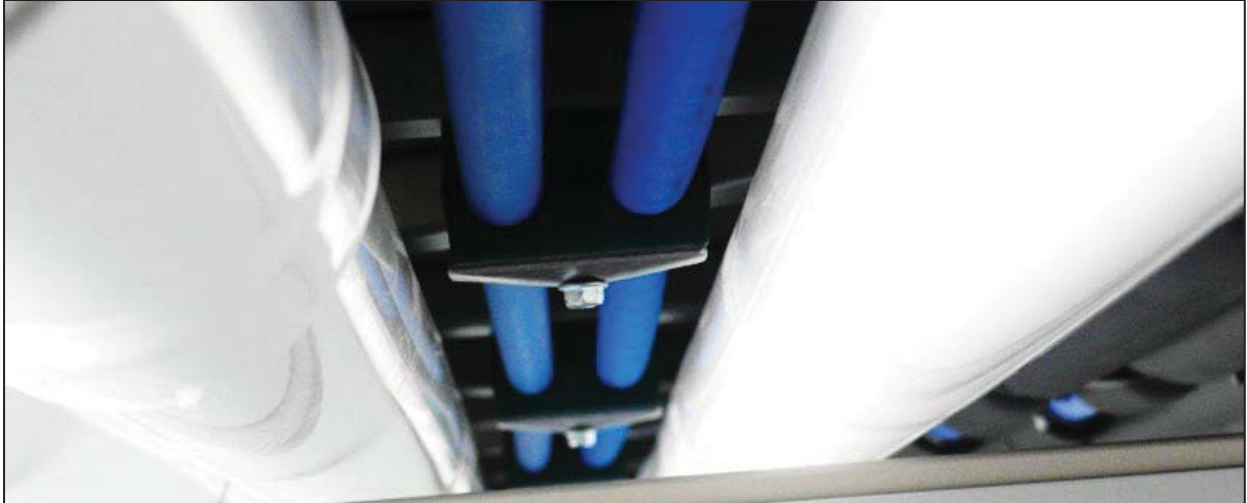
Figure 7: Inside Luggage bays
