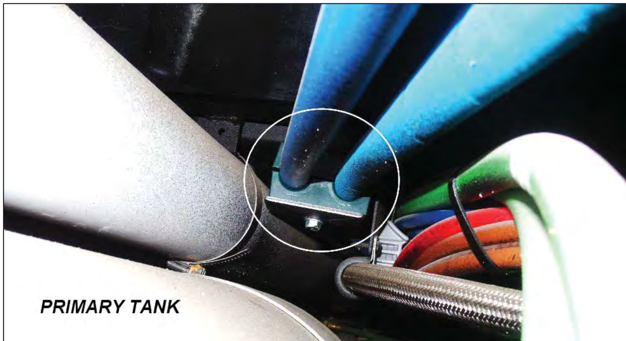
Figure 8: Above Primary Tank Looking Towards the Rear.
