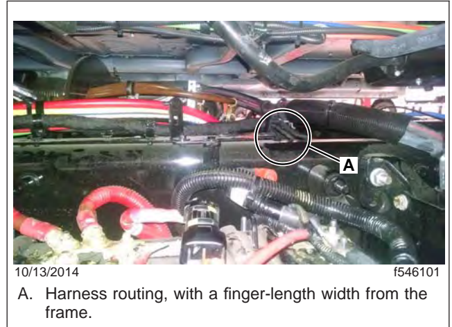
Fig. 2, Aftertreatment Harness Routed Along the Frame
