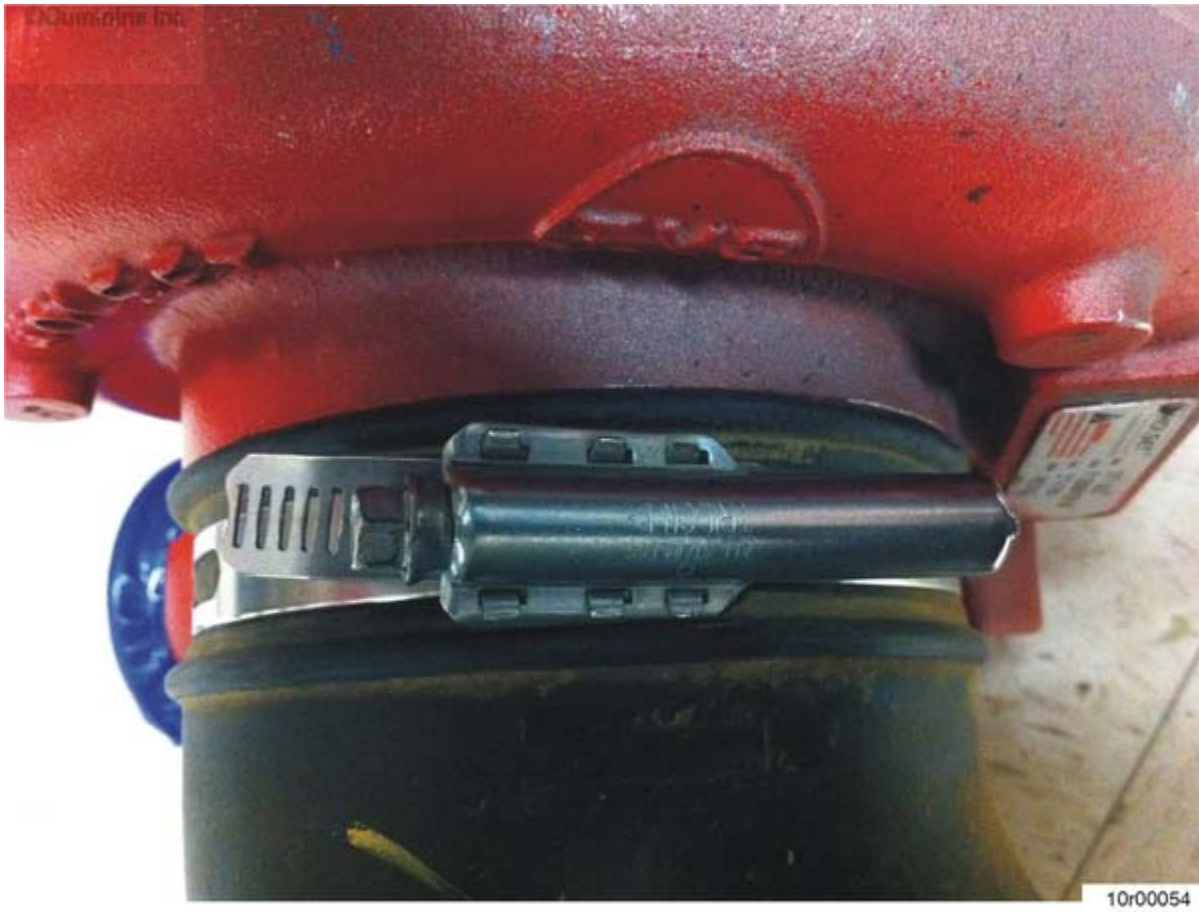
Figure 2: No gap present when clamp is at proper torque.
