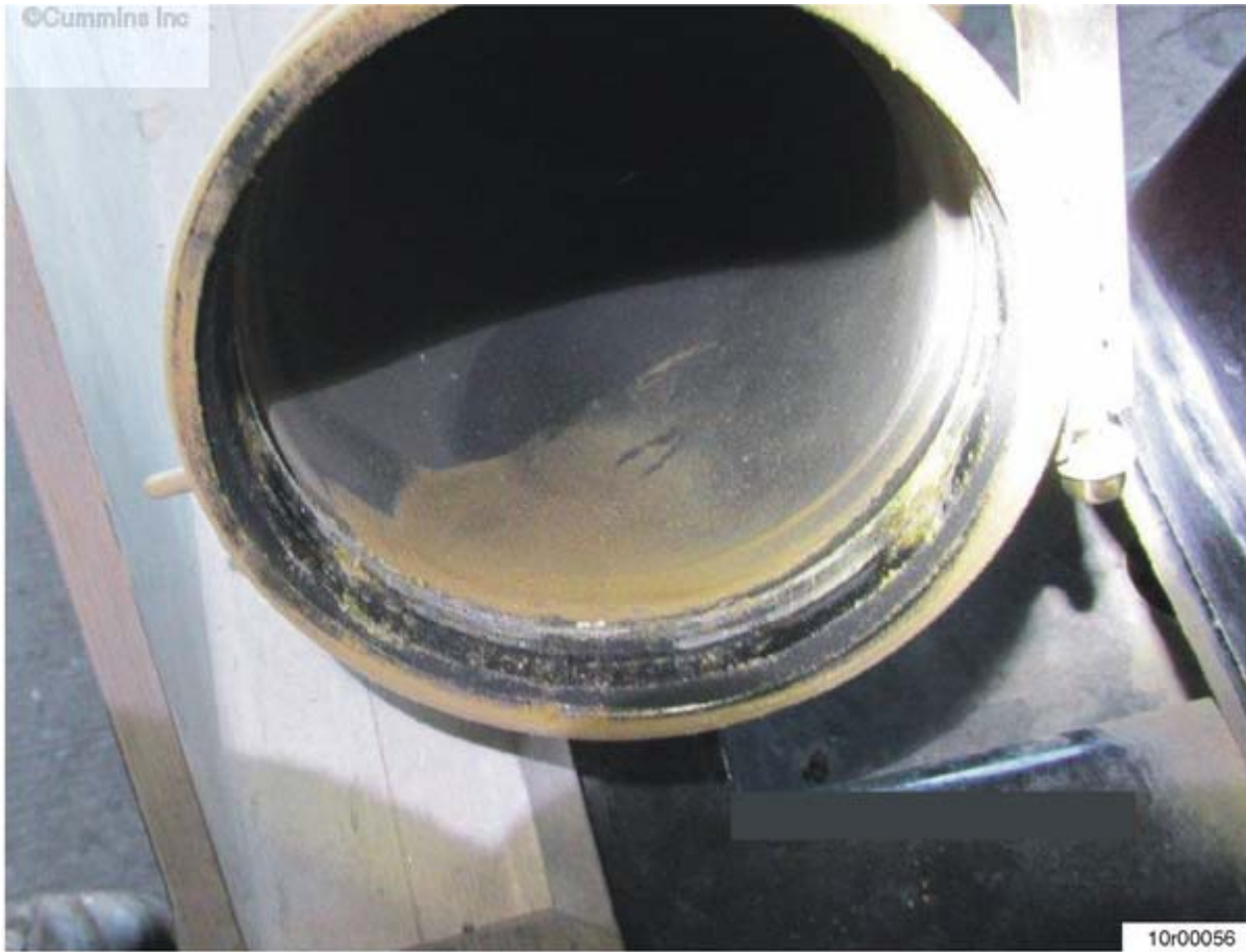
Figure 4: Dust/debris entering the connection point at the turbocharger compressor inlet (the bottom of the hose is the 6 o'clock position).
