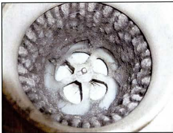
Figure 1. HV Battery Cooling Fan BEFORE Cleaning
