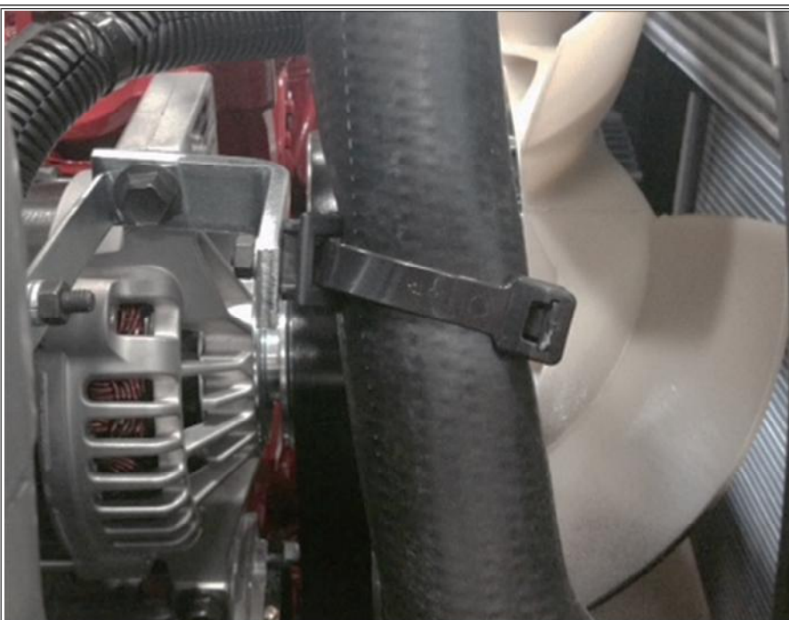
Figure 5: Issues - zip strap over tight, saddle clamp at incorrect angle, and extension bracket at incorrect angle causing saddle and strap to dig into hose
