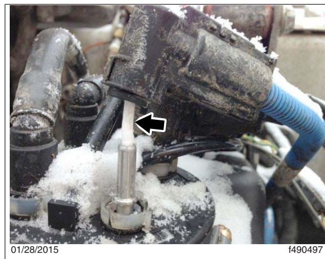
Fig. 1, Ice Expansion at the DEF Line Fitting
