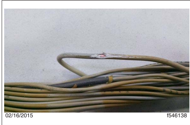
Fig. 1, Worn Insulation, Major
