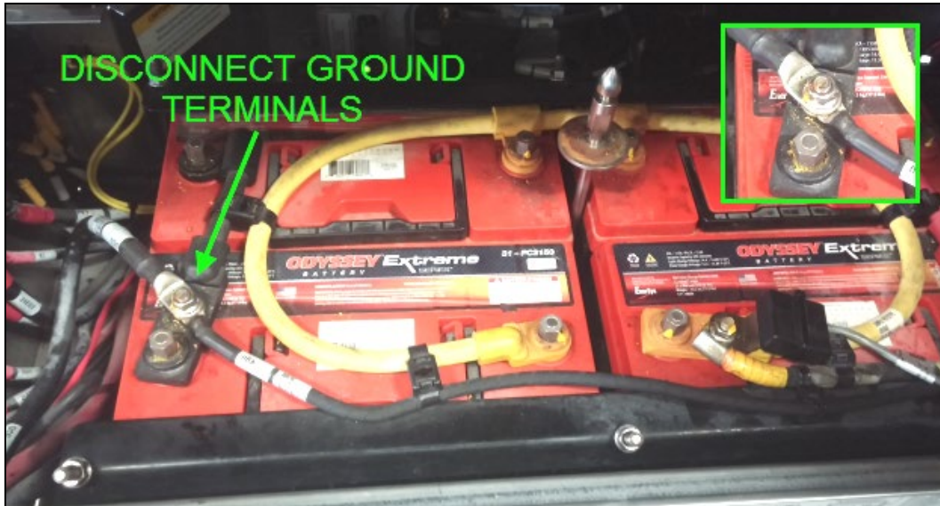
Fig.5 Battery ground terminals to be disconnected first
